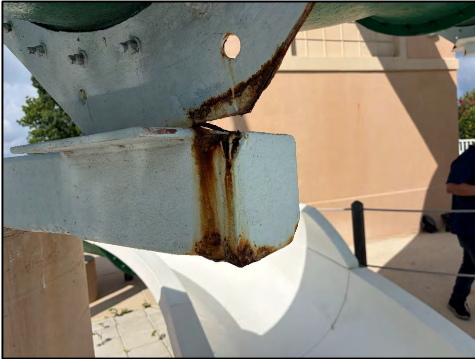
Photo 21 – Support S-5 corrosion at yoke plate.
