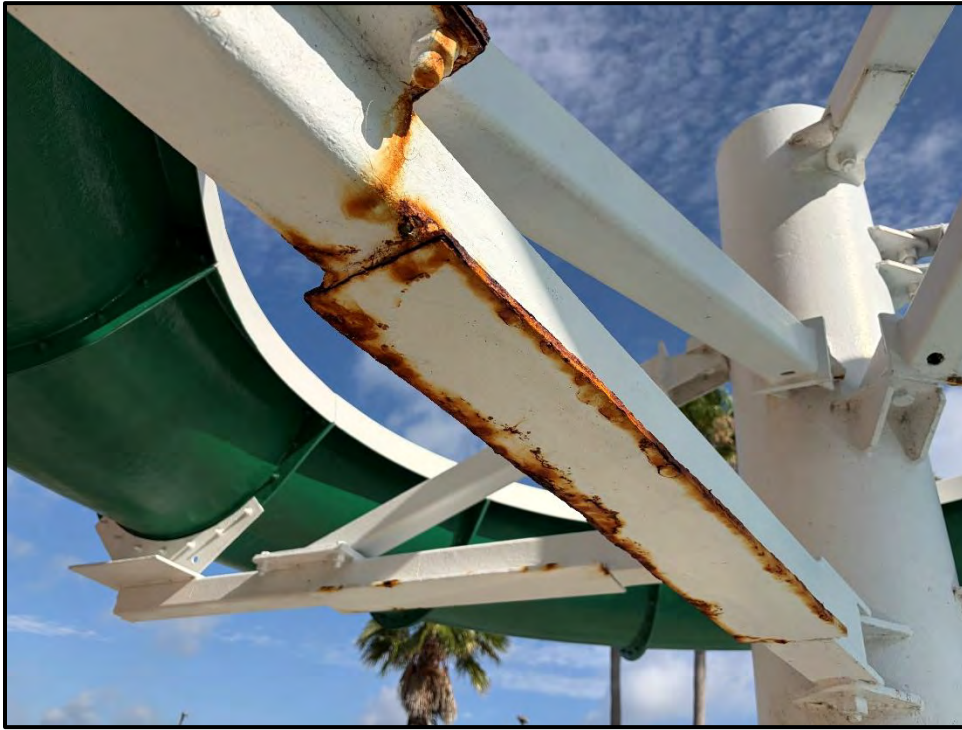
Photo 33– Support PKT-6 beam plate corrosion.
