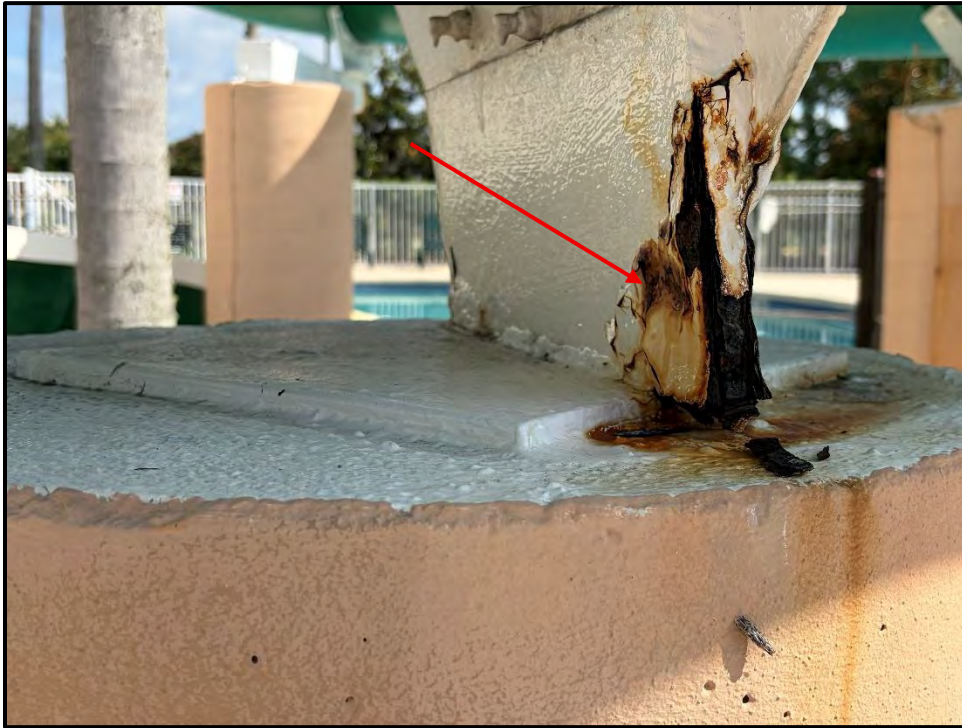
Photo 9 – Support S-3 corrosion on extension plate
