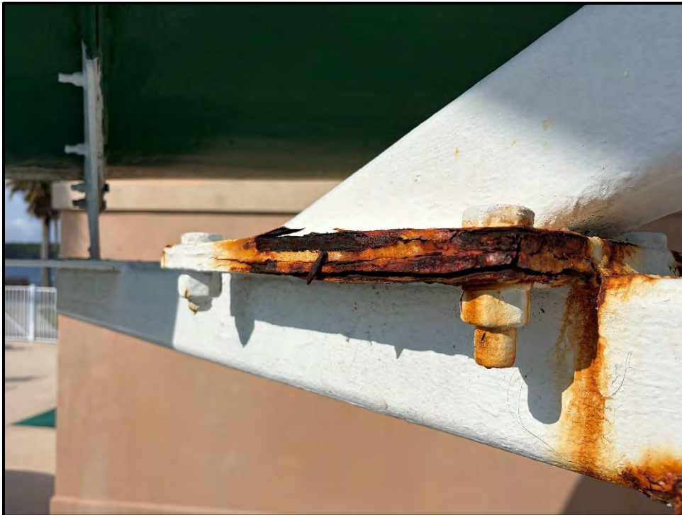
Photo 34– Support PKT-6 bolt plate corrosion.
