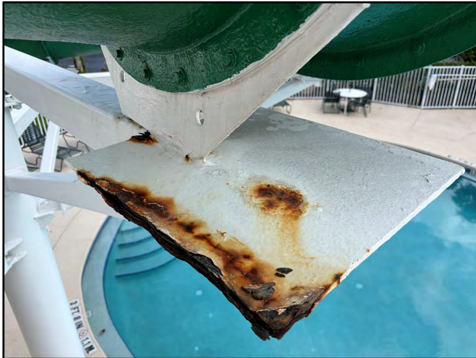
Photo 54 – Support PKT-10 yoke base plate corrosion.
