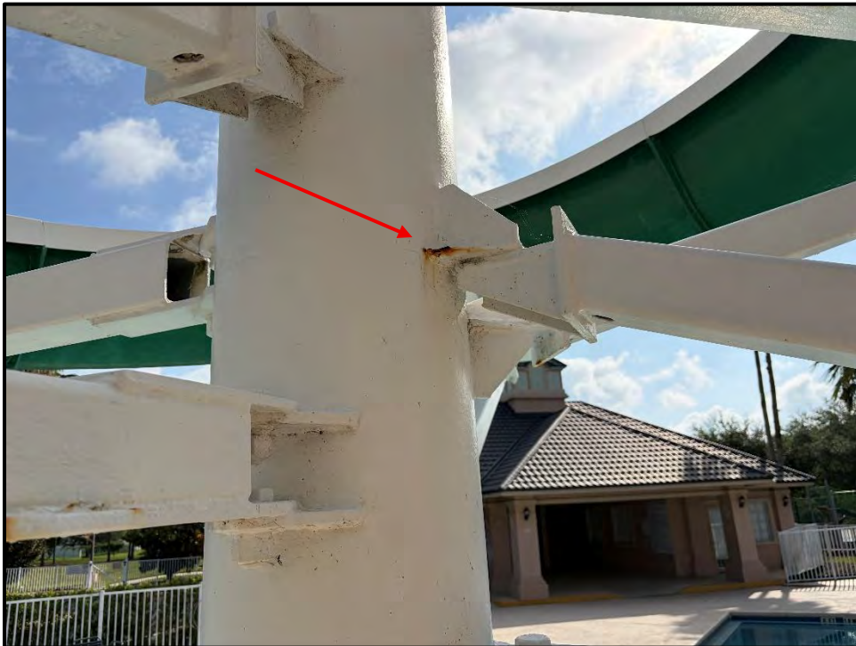
Photo 38– Support PKT-6 column connection corrosion
