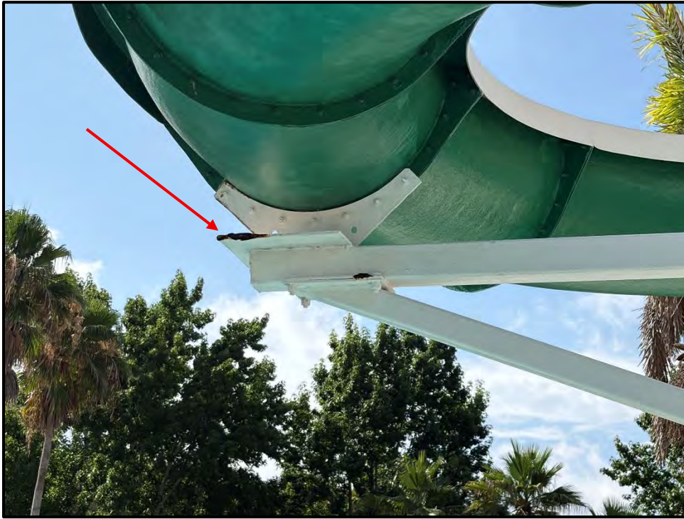
Photo 45 – Support PKT-9 overview. Corrosion observed on the edge of yoke base plate.
