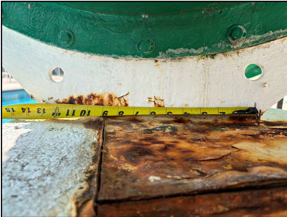
Photo 18 - Support S-4 surface corrosion on base and yoke plate
