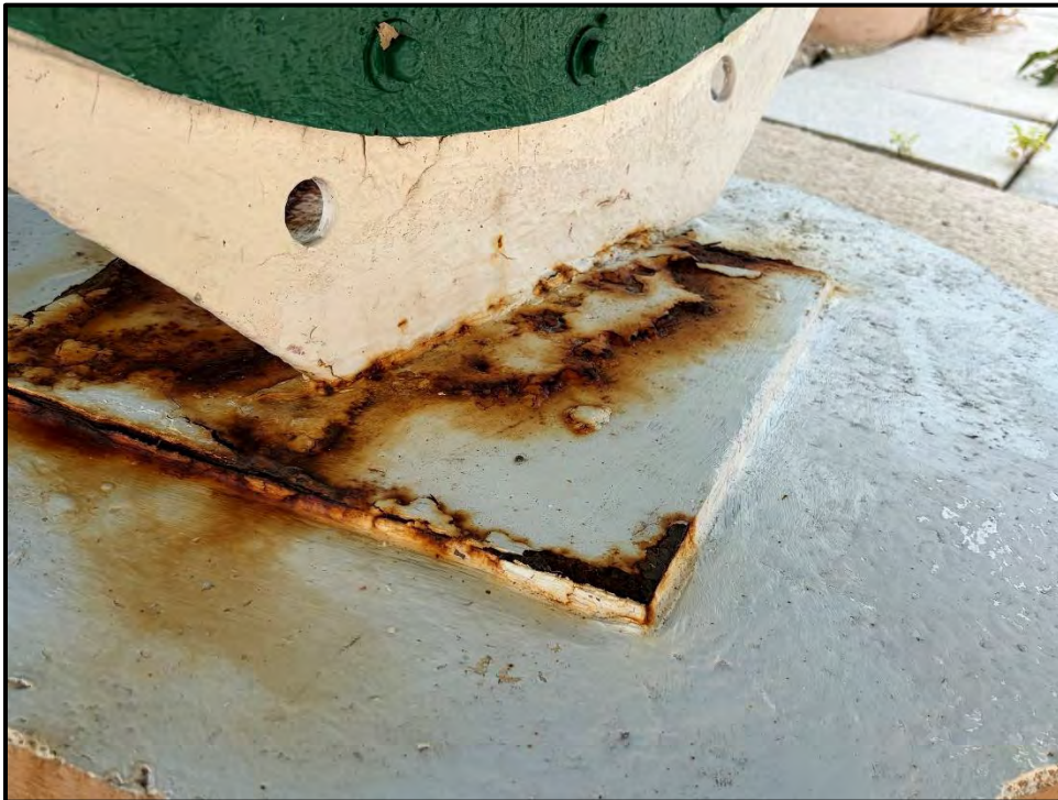
Photo 4 - Support S-1 surface corrosion at baseplate
