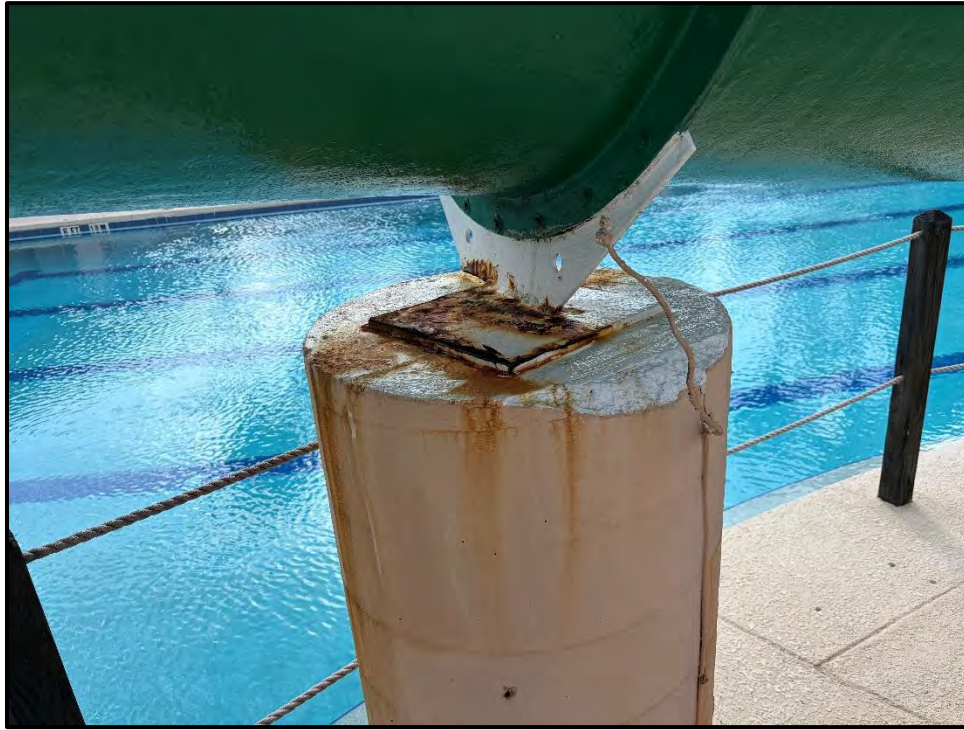
Photo 15 – Support S-4 surface corrosion on base and yoke plate
