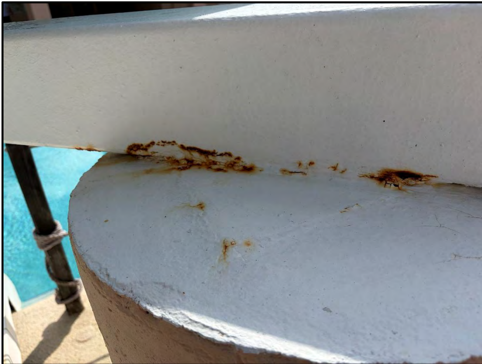
Photo 20 – Support S-5 surface corrosion at baseplate to extension beam connection.
