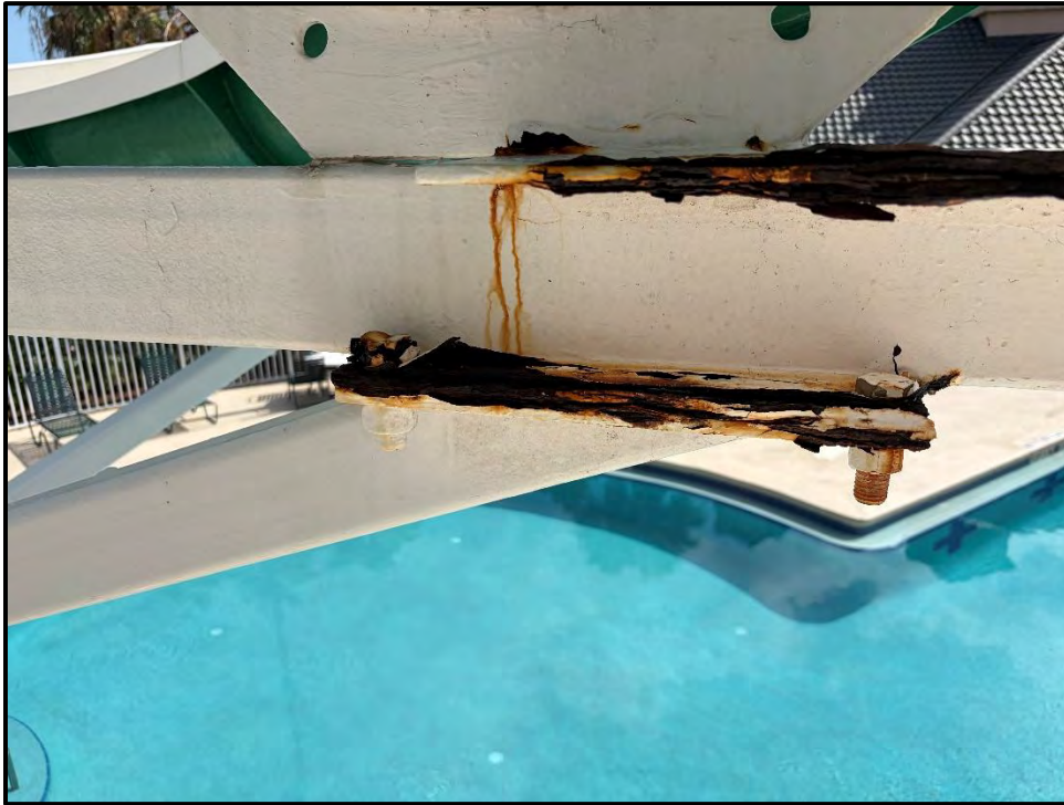
Photo 55– Support PKT-10 bolt plate corrosion.
