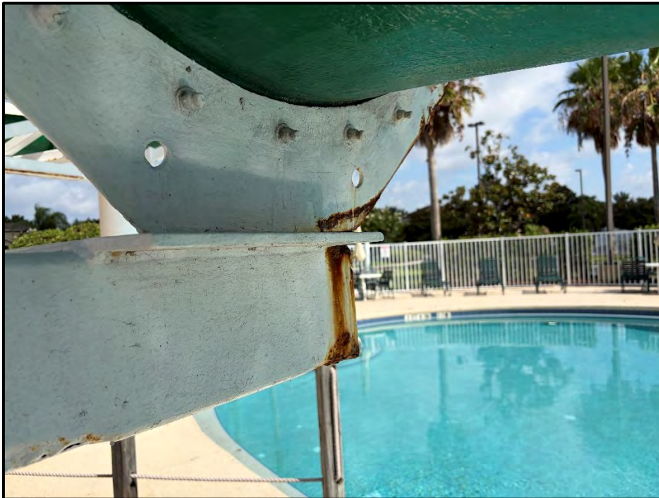
Photo 22 – Support S-5 corrosion at yoke plate.
