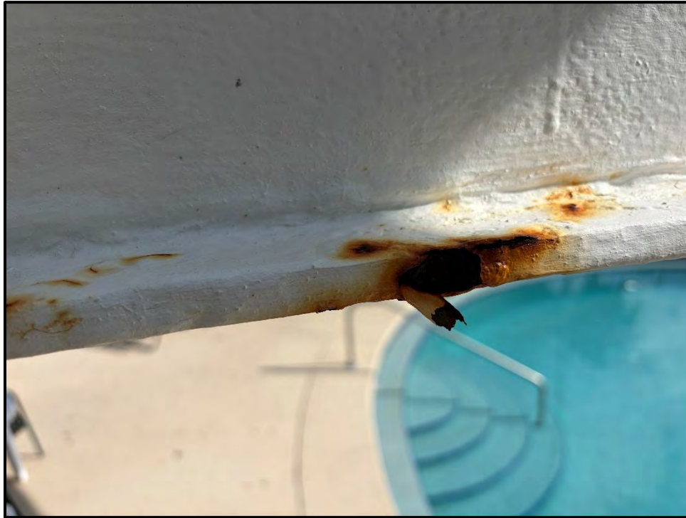
Photo 41– Support PKT-7 beam plate corrosion
