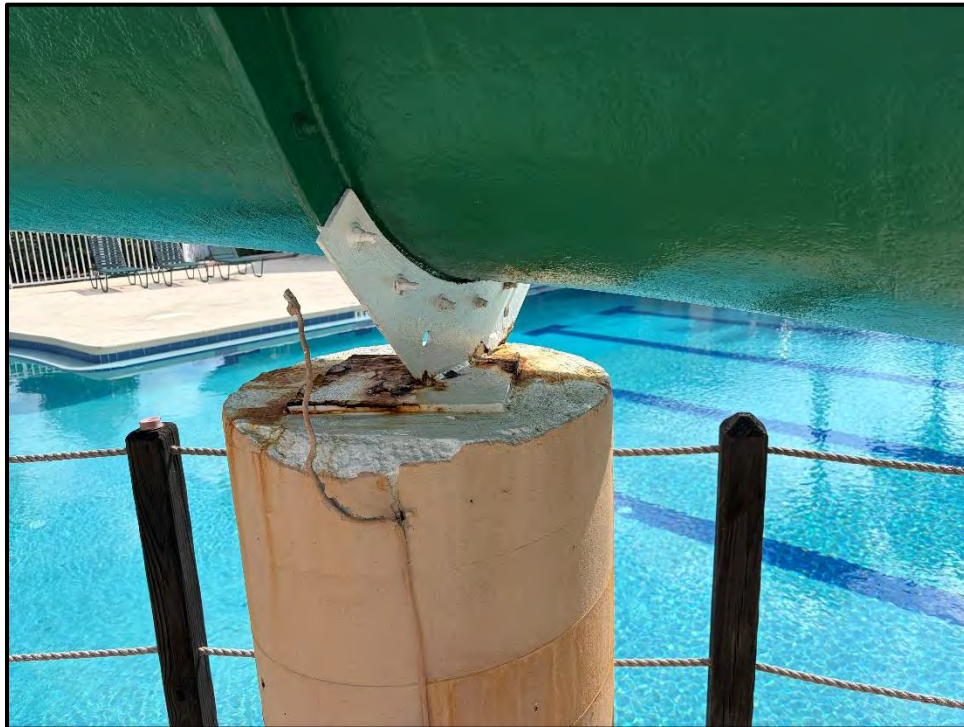
Photo 16 - Support S-4 surface corrosion on base and yoke plate
