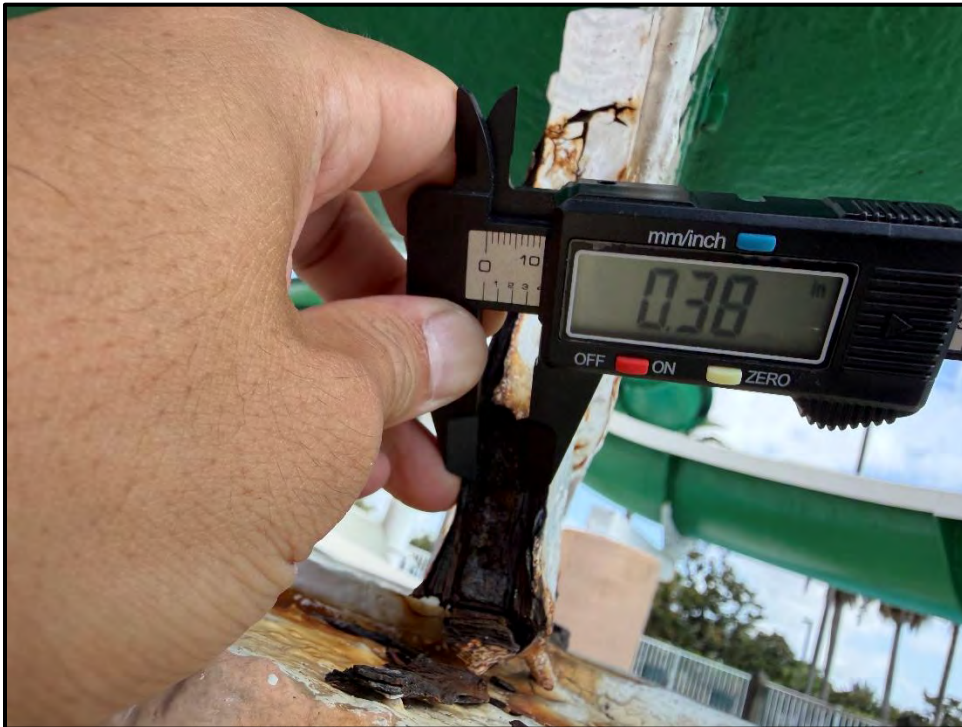
Photo 12 – Support S-3 corrosion on extension plate
