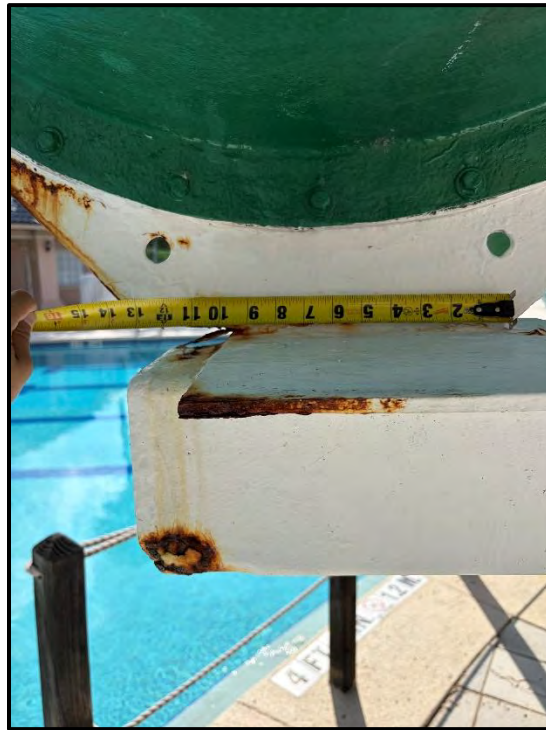
Photo 25 – Support S-5 yoke plate offset from yoke base plate.
