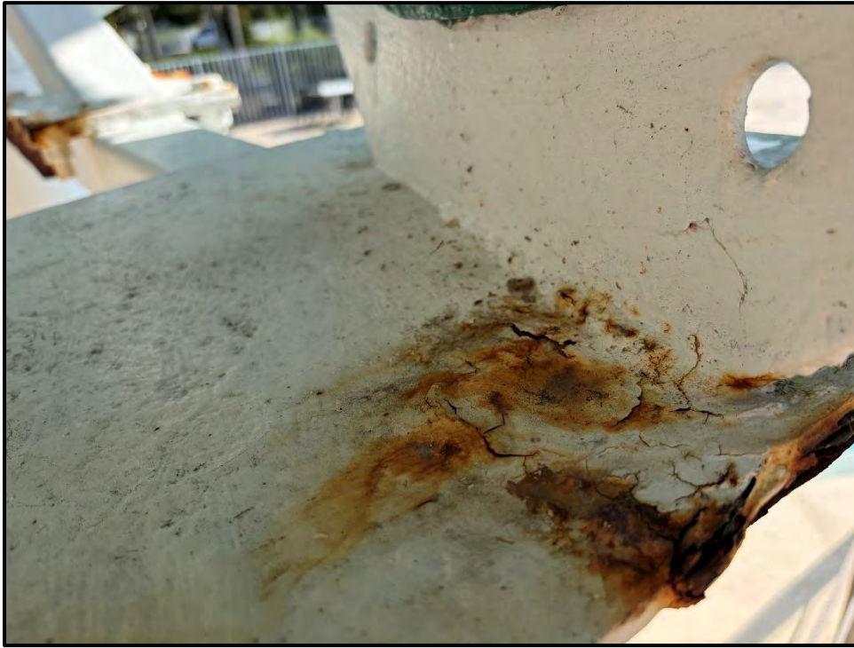
Photo 37– Support PKT-6 yoke base plate corrosion
