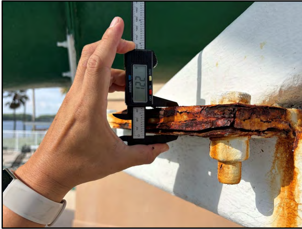
Photo 35– Support PKT-6 bolt plate corrosion.
