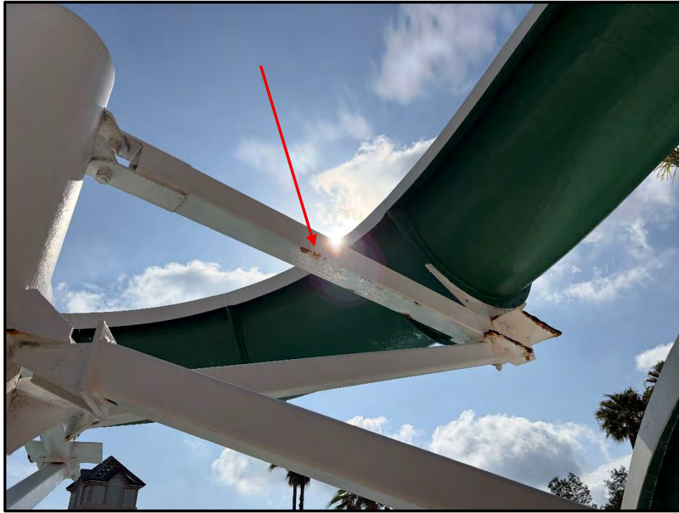
Photo 51 – Support PKT-10 overview. Beam surface corrosion observed.
