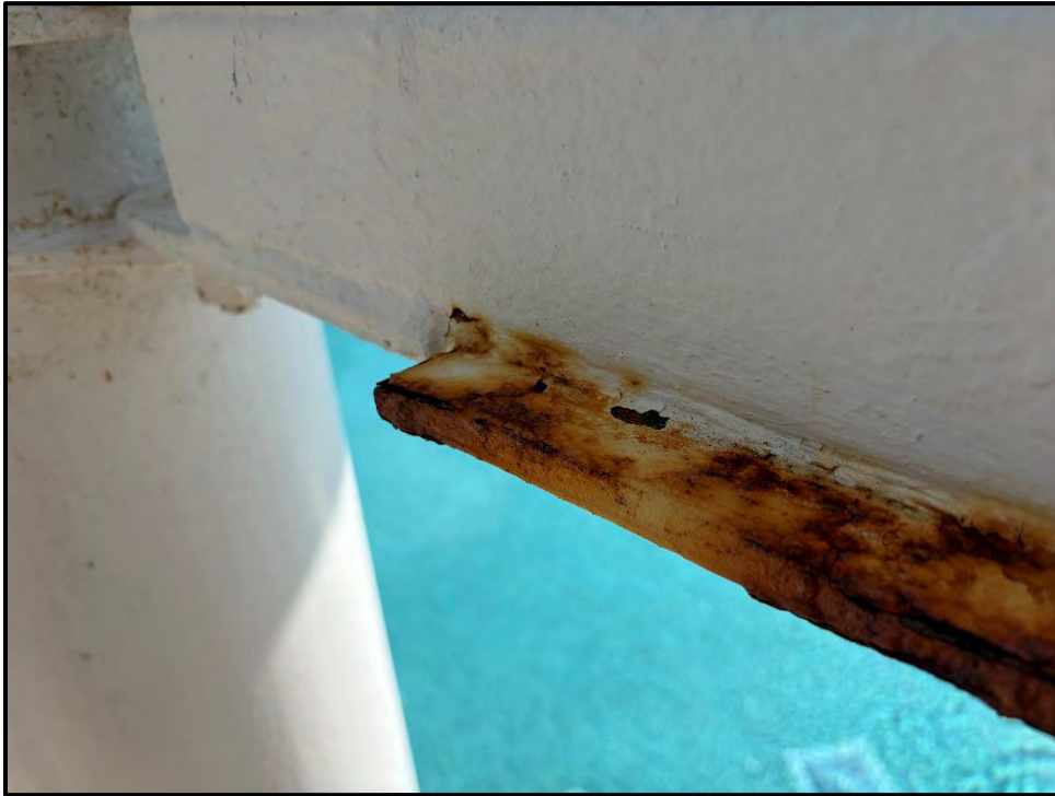
Photo 27 – Support PKT-6 beam plate corrosion.
