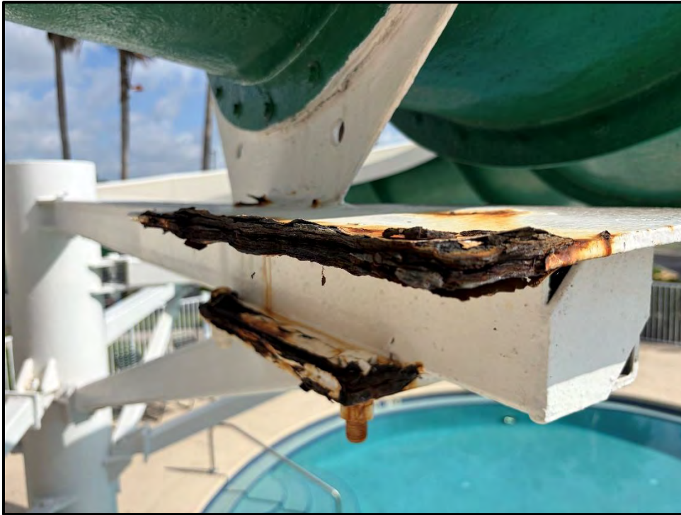
Photo 57– Support PKT-10 bolt plate and yoke base plate corrosion.
