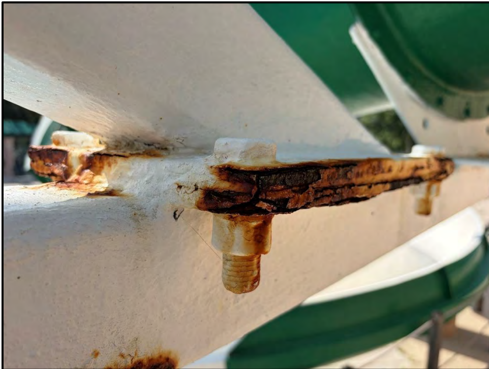
Photo 32– Support PKT-6 bolt plate corrosion.
