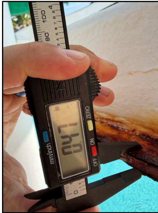
Photo 29– Support PKT-6 beam plate corrosion.
