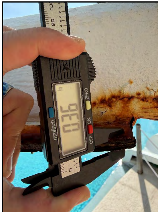
Photo 30– Support PKT-6 beam plate corrosion.
