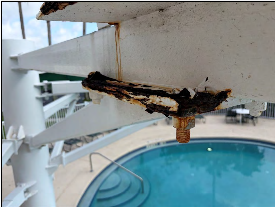
Photo 58 – Support PKT-10 bolt plate corrosion.
