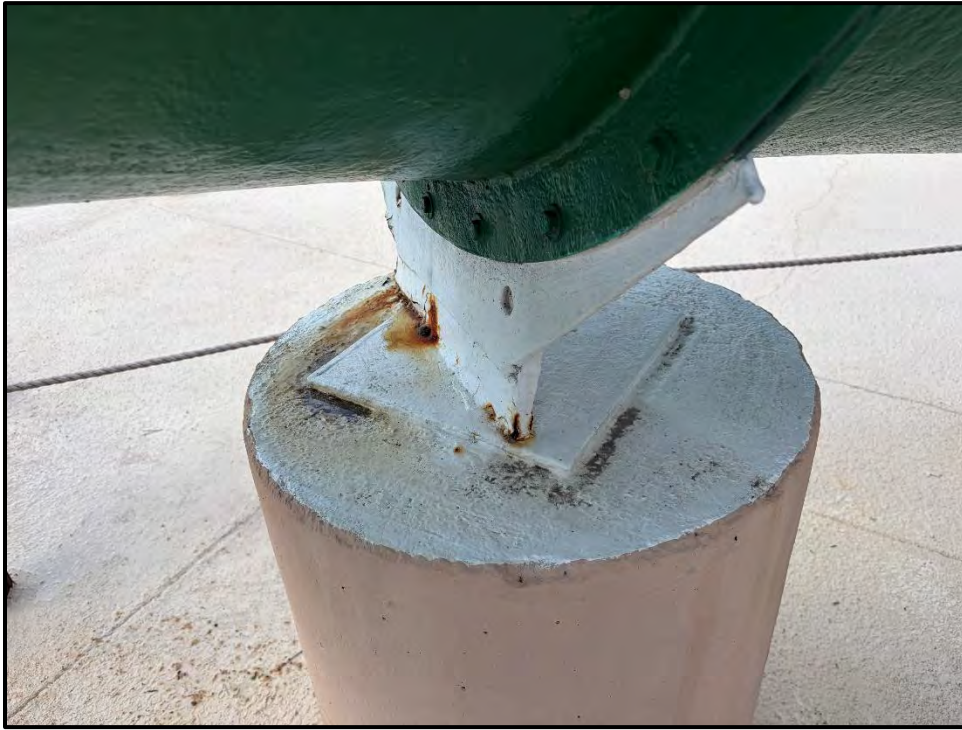
Photo 13 – Support S-3 corrosion on extension plate
