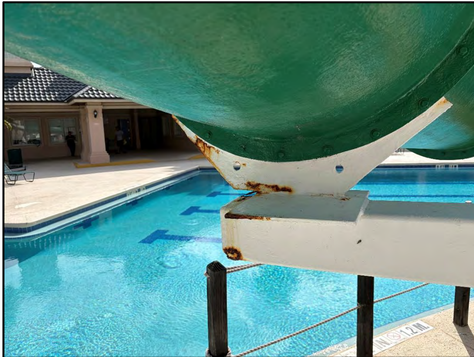
Photo 24 – Support S-5 surface corrosion at yoke and yoke base plate.
