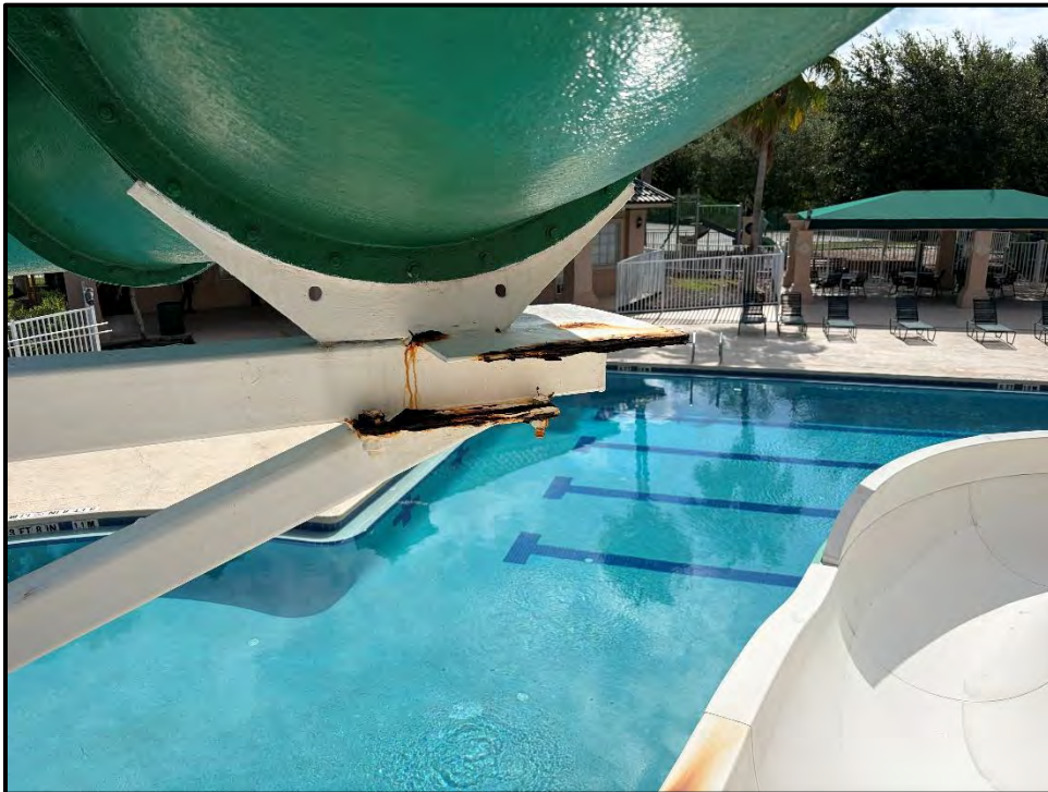
Photo 56– Support PKT-10 bolt and yoke base plate corrosion.
