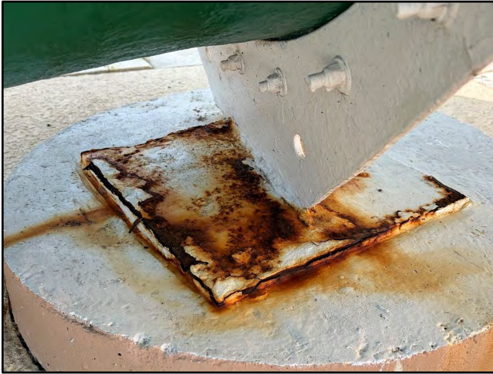
Photo 3 – Support S-1 surface corrosion at baseplate
