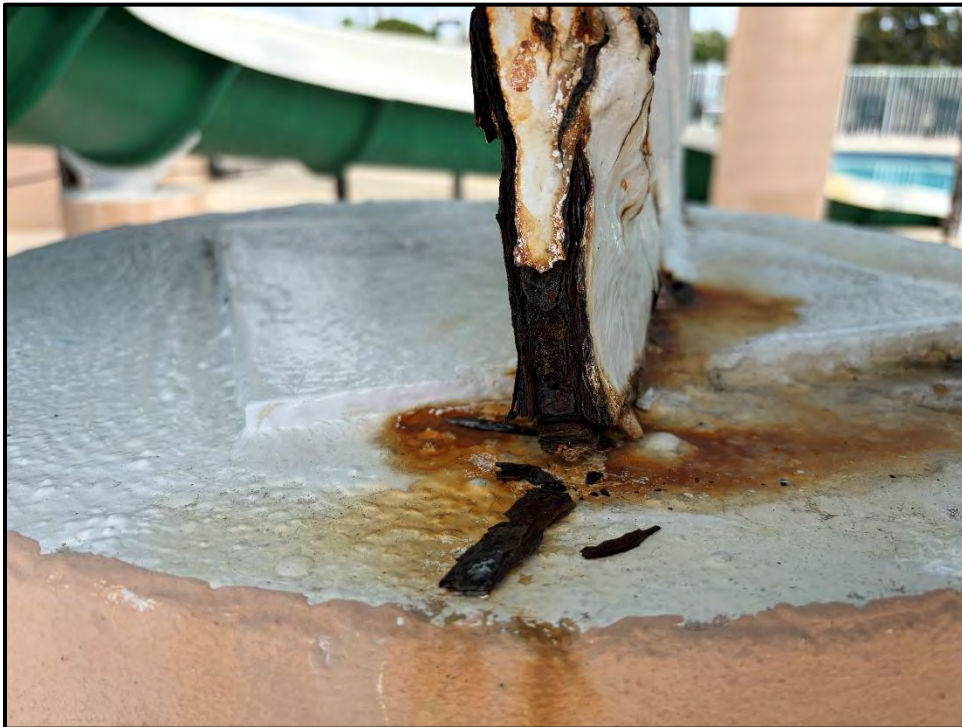
Photo 10 – Support S-3 corrosion on extension plate
