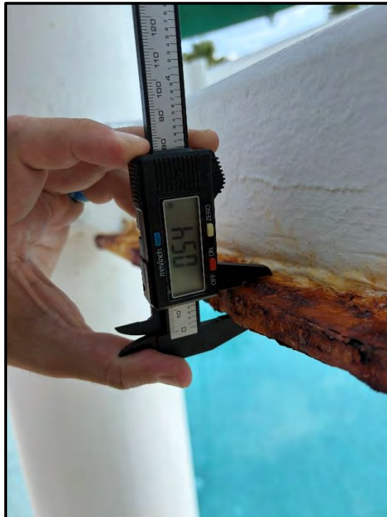
Photo 28– Support PKT-6 beam plate corrosion.
