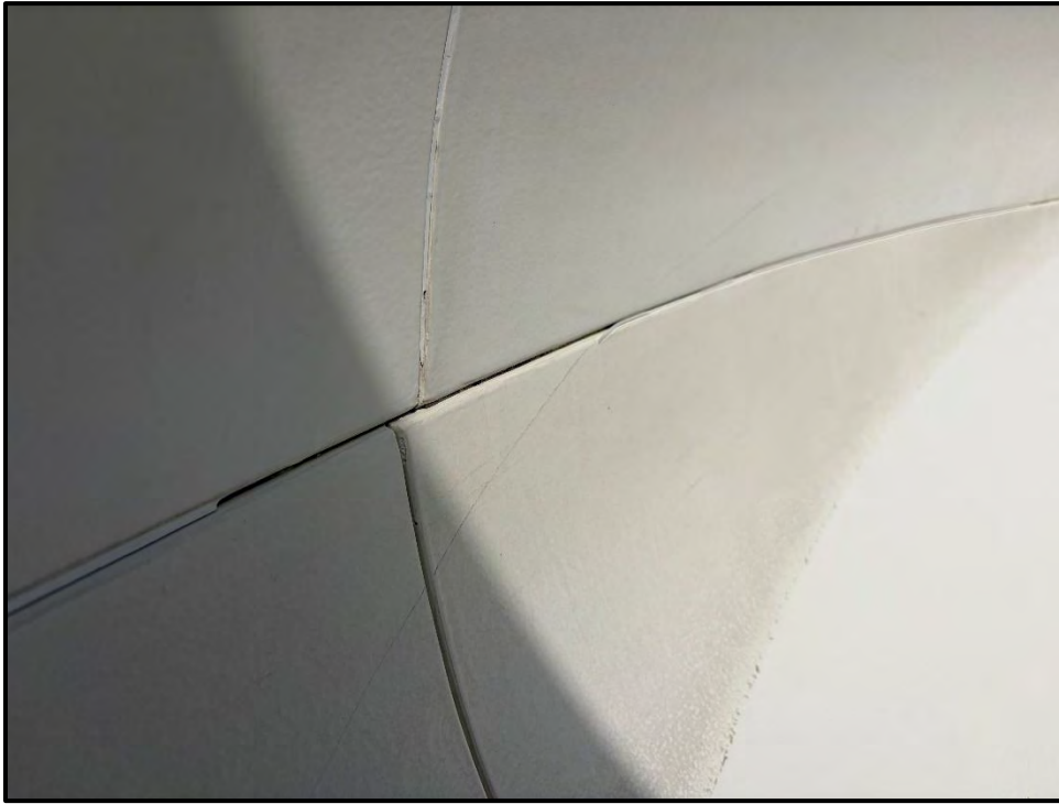
Photo 59 – Typical slide seam gaps .
