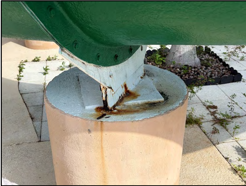
Photo 11 – Support S-3 corrosion on extension plate
