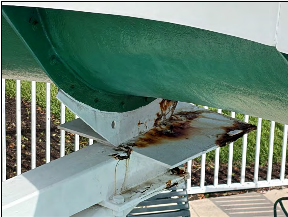
Photo 44– Support PKT-8 yoke and yoke base plate corrosion.
