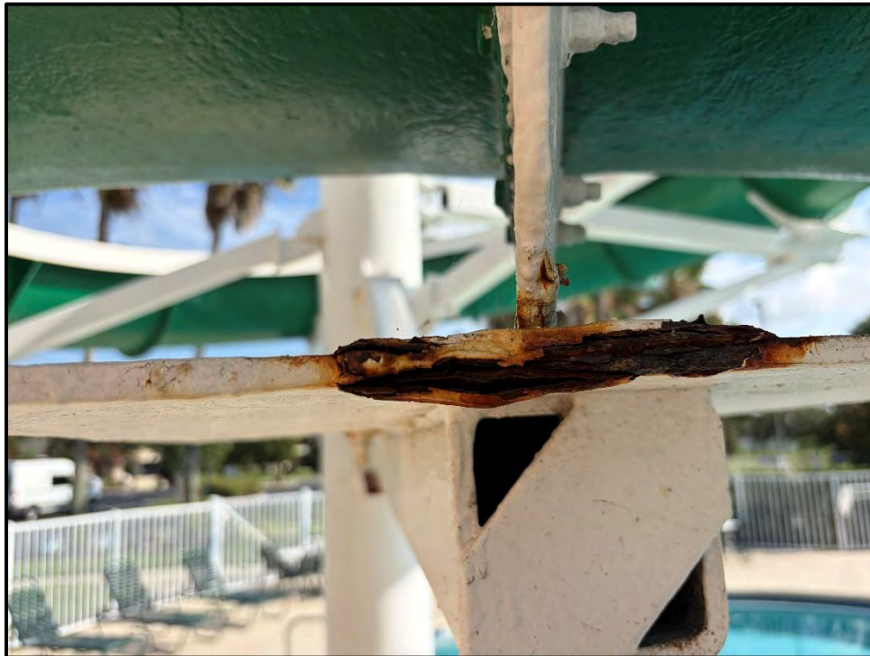
Photo 36– Support PKT-6 yoke base plate corrosion.
