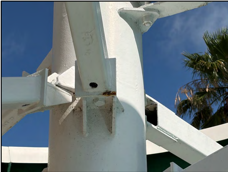
Photo 50 – Support column plate connection to PKT-10 showing surface corrosion.
