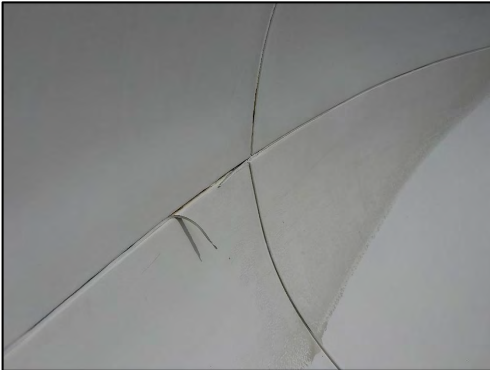
Photo 60 – Typical slide loose joint sealant.
